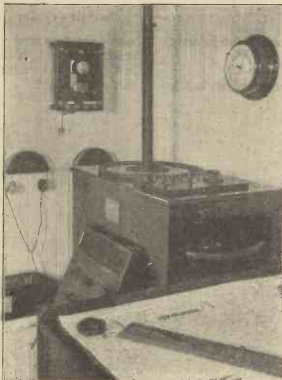
Complete Direction Finder Equipment installed in Chart Room, S.S. "Cairnross" (Messrs. Cairns, Noble & Co.).
